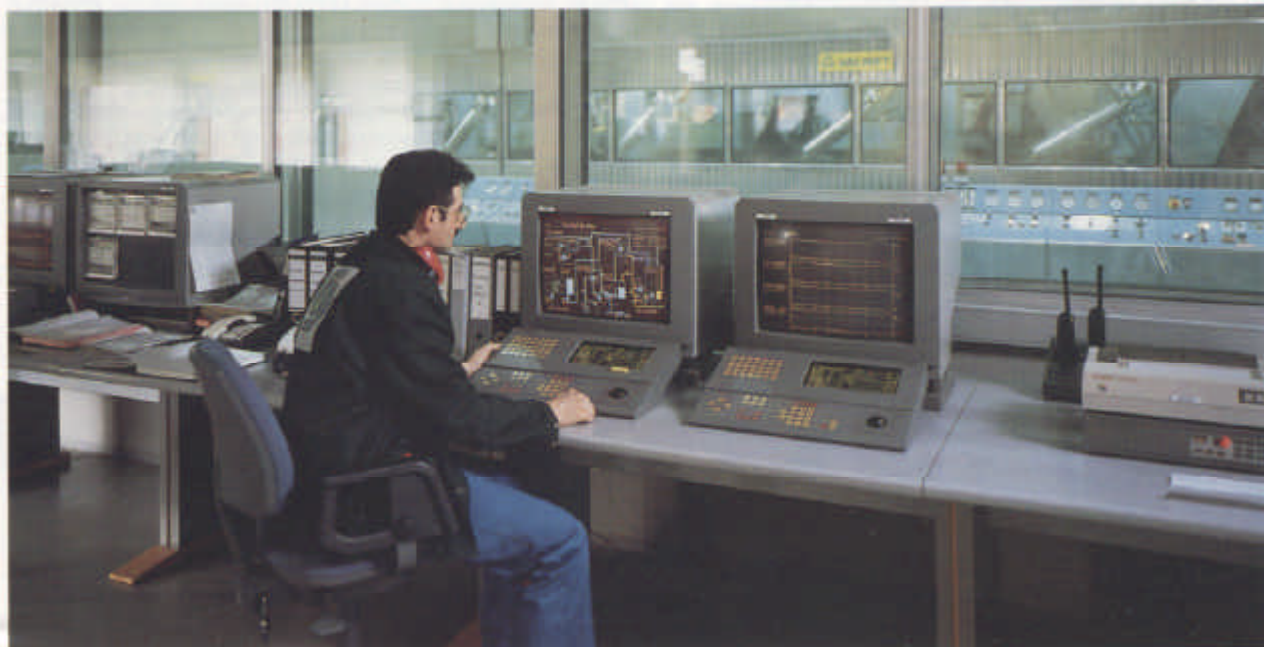
One of the Damatic XD control rooms
